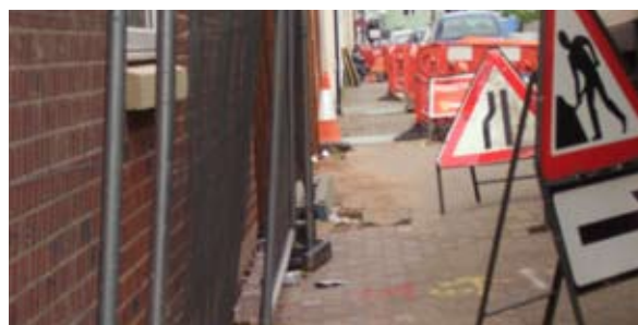
A photograph showing hazards in a road near a school, taken by children conducting a safety audit
